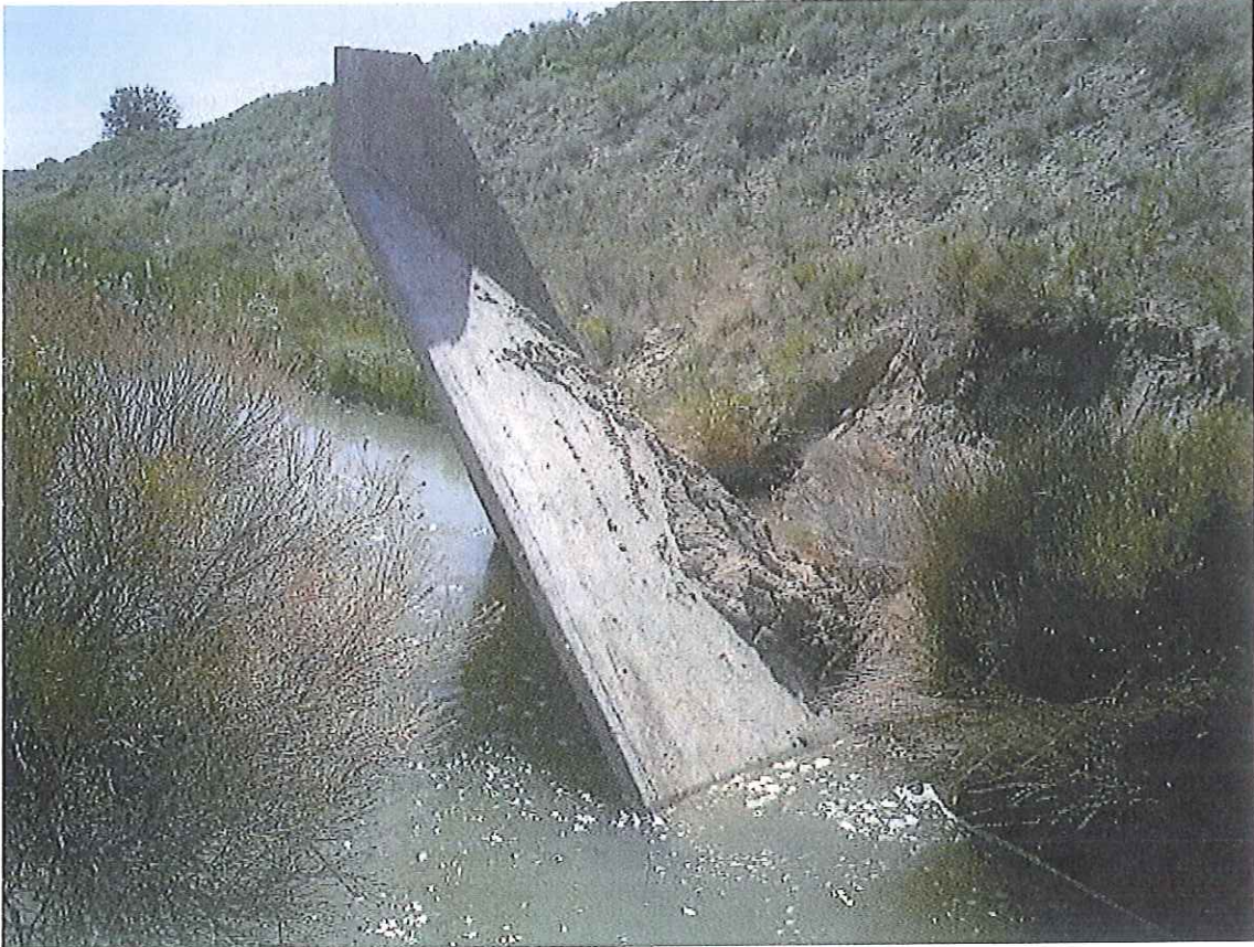
FAILED CONCRETE DROP STRUCTURE APRON
