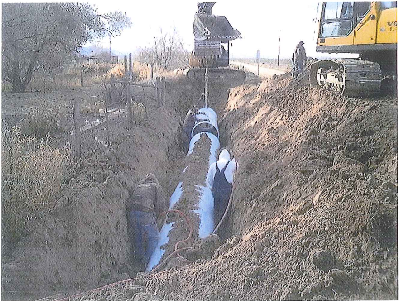
Wyoming Canal 15.1 Lateral-36 inch diameter PVC pipe
