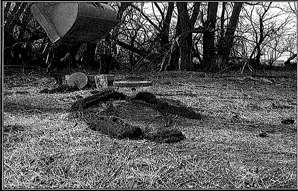
TREE ROOTS REMOVED FROM UNDERGROUND DRAIN
