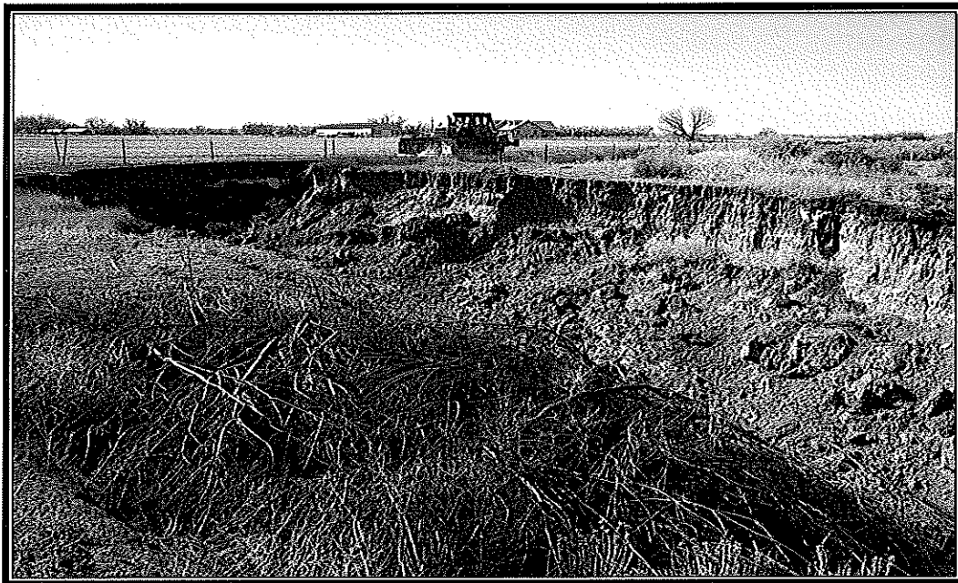
WASHOUT CAUSED BY WASTE WATER
